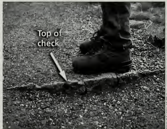
Fig. 6-10 After approximately three years, there is slight erosion of the tread, but no gullying is present on the Ocean Path (#3).
