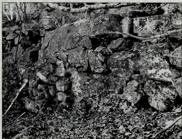
Fig. 6-33 This retaining wall on the Gurnee Path (#352) is rubble at the bottom and laid at the top.
