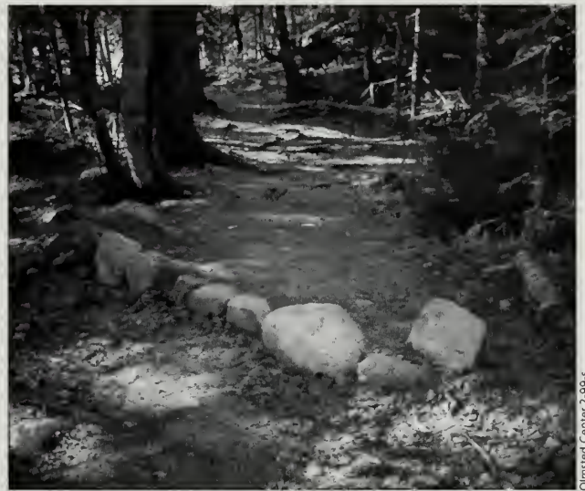
Fig. 4-39 A recently constructed stone water bar on the Pond Trail (#20), located between the motor road and the Jordan Pond Path (#39).
