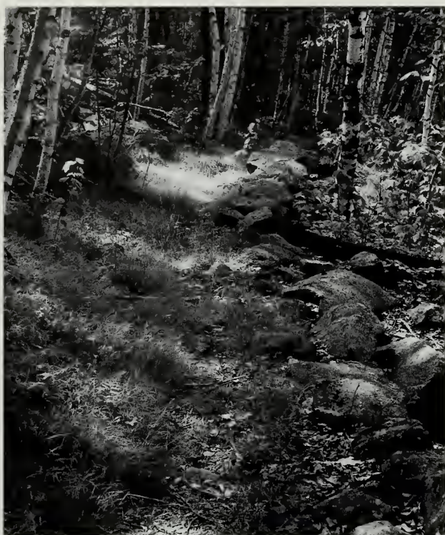
Fig. 6-31 A classic example of original coping retaining wall on the Wild Gardens Path (#354) using large single boulders for retention.
