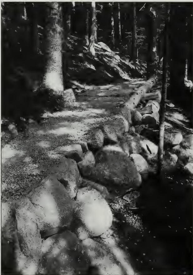
Fig. 6-55 Wall crib on steepest west-side section of the Jordan Pond Path (#39) built in conjunction with stone retaining wall.
