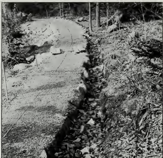
Fig. 4-36 A walled side drain installed on the Jordan Pond Path (#39) along new walled causeway in 2001. Temporary wood planks cover the new open stone culvert.
