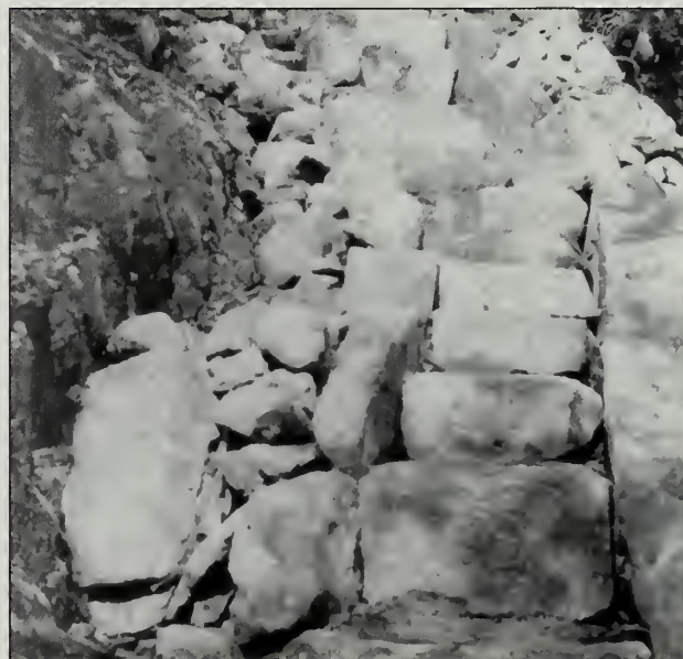
Fig. 4-29 A circa 1935 photograph of a CCC rehab of the lower section of the Ladder Trail (#64) shows a rubble French drain being installed along the side of a staircase with coping retaining wall.
