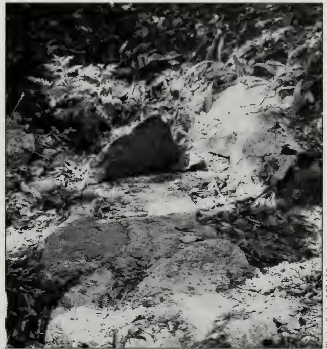
Fig. 4-16 Located near the base of the Perpendicular Trail (#119), a small CCC graveled-over culvert now has underlying capstones visible due to loss of gravel. A catch basin (difficult to discern in the photo) is in the foreground and a coping stone is visible on far side of treadway.
