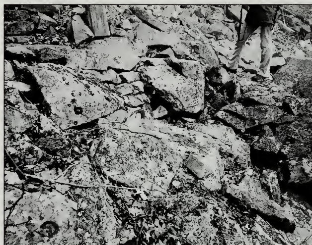
Fig. 6-34 Fitted retaining wall built into the talus slope on the Champlain Mountain East Face Trail (#12).
