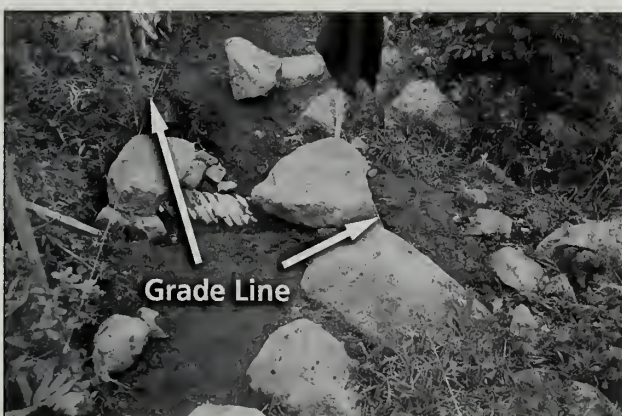
Fig. 4-4 A new 2002 pipe culvert on Jordan Pond Path (#39). The photo shows header stones before crush and gravel surfacing, which will completely cover the pipe. Note lintel stones meet grade line at outside edge.
