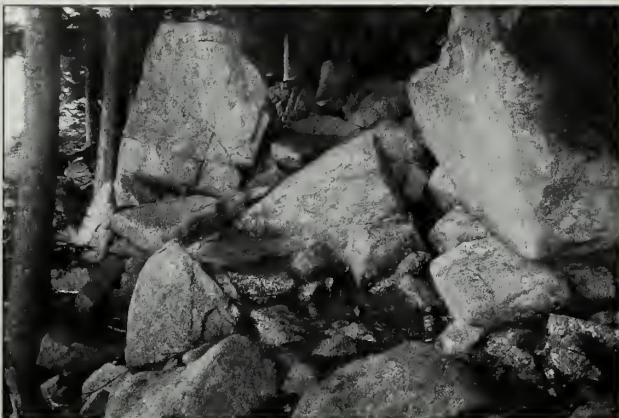
Fig. 7-42 Dilapidated Bates-style steps on the Jordan Pond Path (#39) before NPS rehabilitation, see Fig. 7-43.
