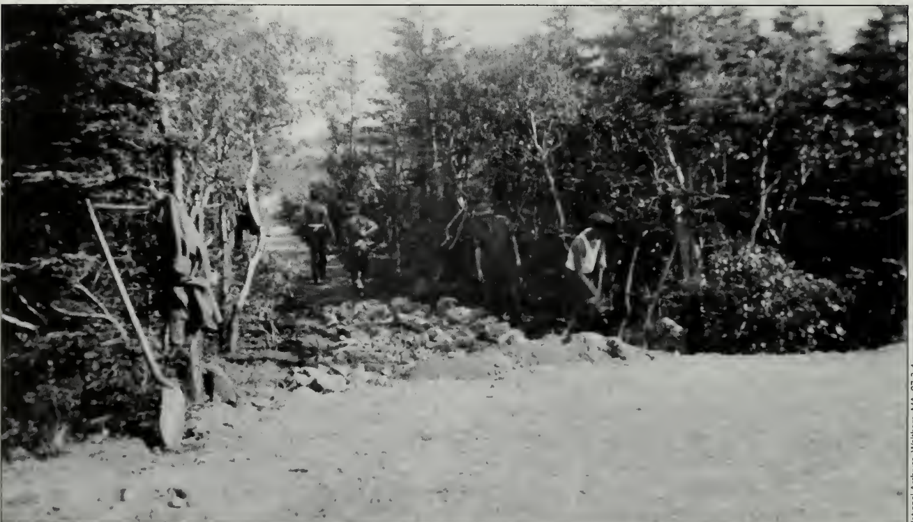
Fig. 3-29 The CCC usually installed rubble base under their gravel tread, work in progress in the 1930s.
