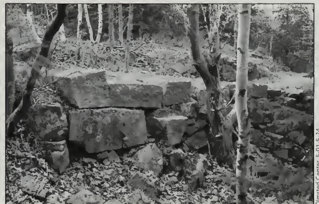
Fig. 6-39 This Mission 66 retaining wall on the Anemone Cave Trail (#369) consists of laid wall upon a rubble wall base.
