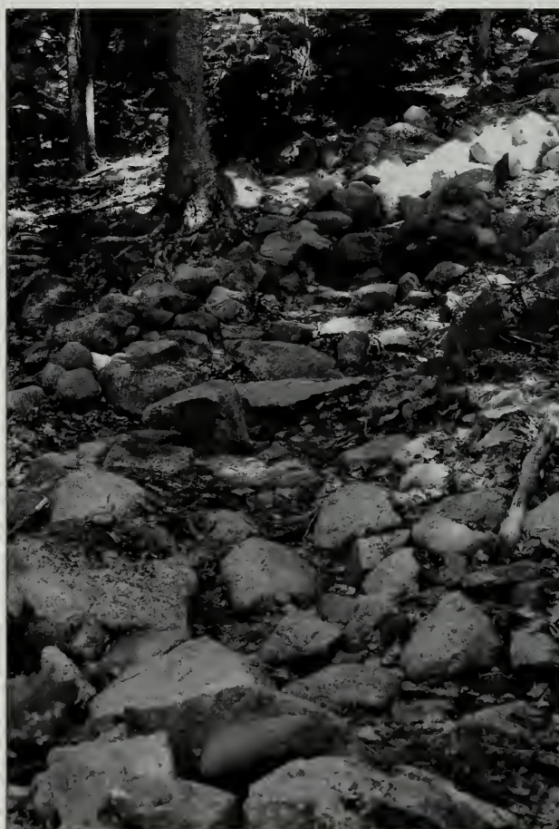
Fig. 7-39 These AMC-style steps on the Pond Trail (#20) were built according to AMC handbook. However, this style of step work, with uneven, slanted steps and the heavy use of scree, is not appropriate for the Acadia trail system.
