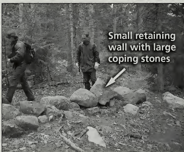
Fig. 6-13 This section of coping retaining wall has larger coping stones atop a relatively small wall on the Asticou Trail (#49).
