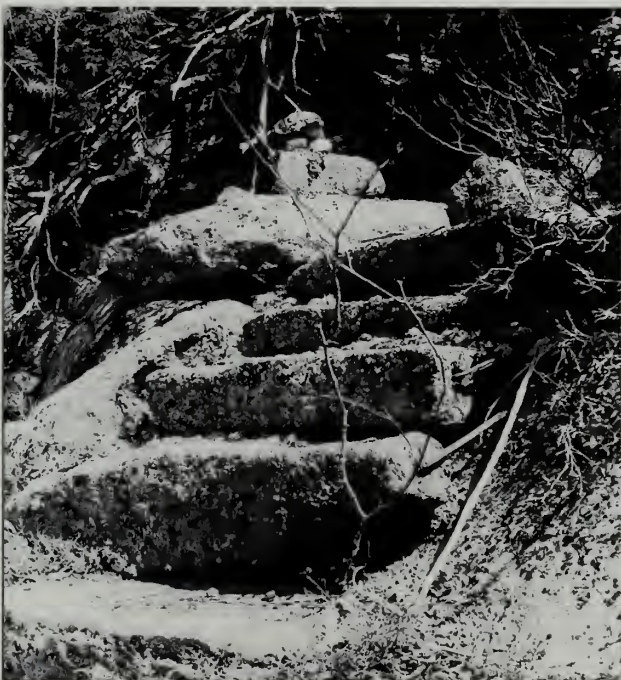
Fig. 8-23 An unusual placement of pins holding steps on the Van Santvoord Trail (#450).
