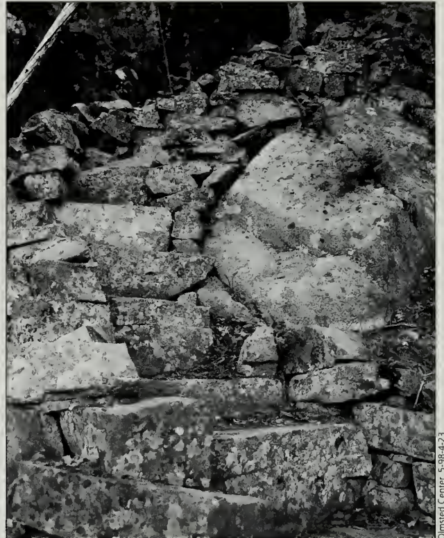
Fig. 8-34 This section of coping and retaining wall along a staircase on the Perpendicular Trail (#119) is held in place with iron pins that are expertly hidden among the stone. It is typical of the type of ironwork used by the CCC on this trail.
