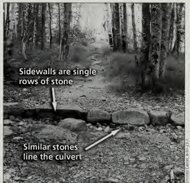
Fig. 4-5 A recently constructed open stone culvert on the Jesup Path (#14) with walls of single stones. This is not an appropriate culvert style for a trail that historically contained graveled-over stone culverts and wooden bridges.
