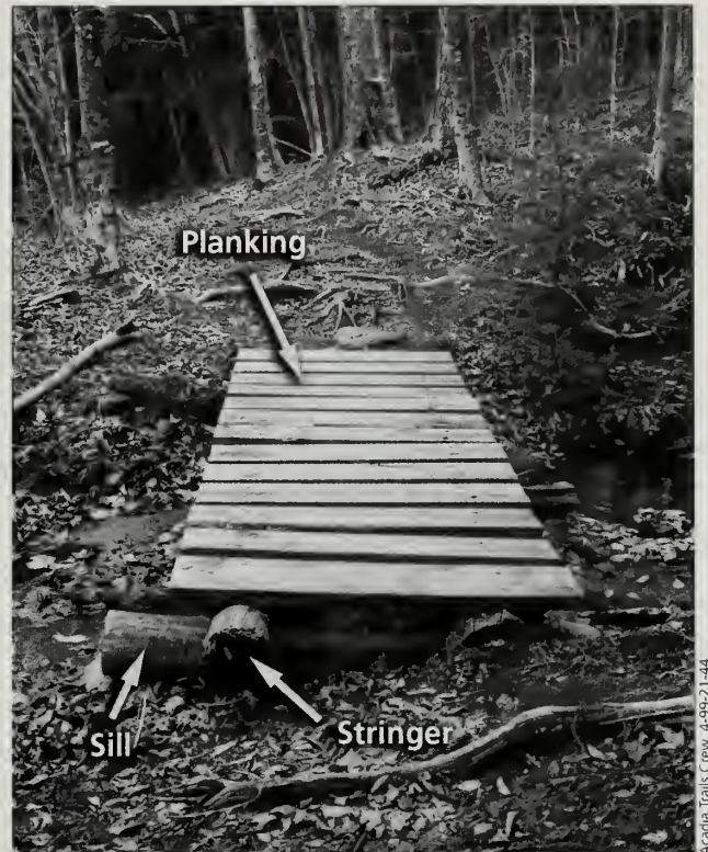
Fig. 5-14 A bridge constructed by the Youth Conservation Corps on the Jordan Pond Carry Path (#38) in 1987.
