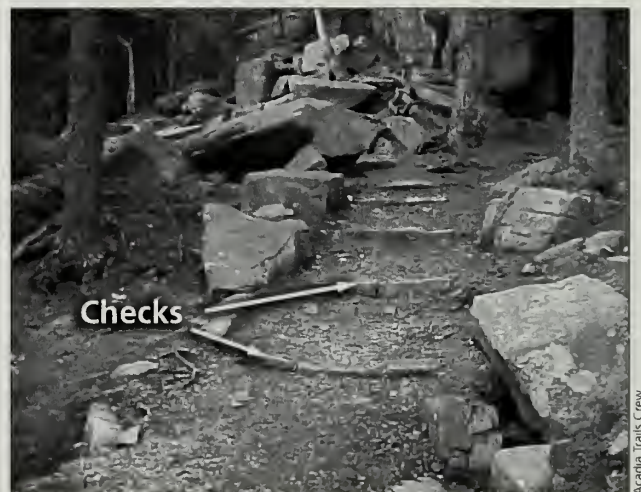
Fig. 6-2 Although a standard feature in other trail systems, particularly in the Western parks, checks have only been used at Acadia since 1995 when these were first installed on the Ocean Path (#3). The slope at this location is approximately 15 percent, and after five years there has been a loss of approximately 3 inches of tread material.
