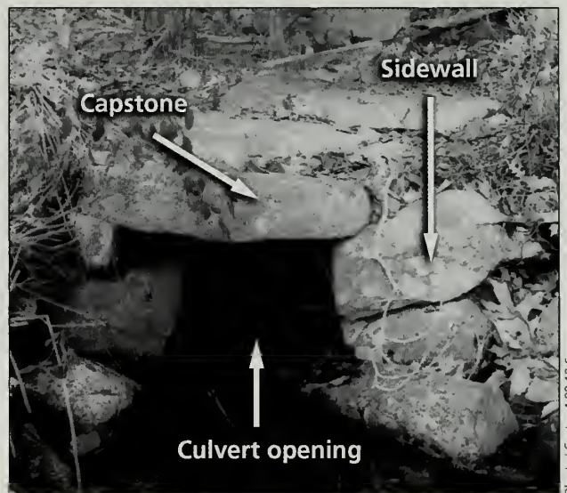
Fig. 4-2 A graveled-over culvert on the Kane Path (#17). The lintels were once completely covered with gravel and vegetation.
